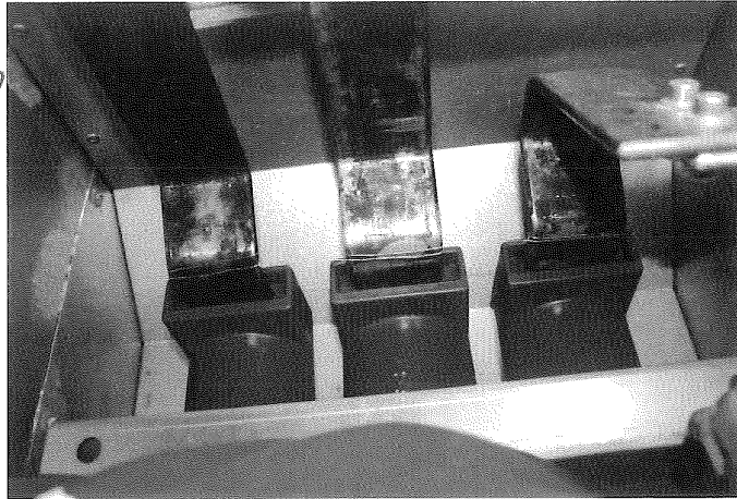
Photo No. 05 Before test PEHLA 11202Ra / 03
