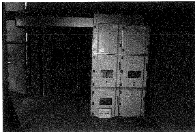
Photo No. 02 Before test PEHLA 11203Ra / 03
