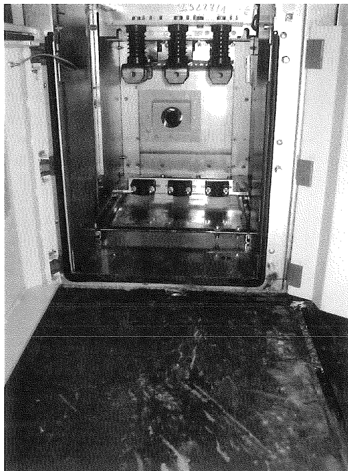
Photo No. 03 Before test PEHLA 11202Ra / 03
