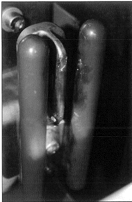
Photo No. 03 After PEHLA 08008Ra / 09 (fixed contact of phase L1, all contacts in comparable condition)
