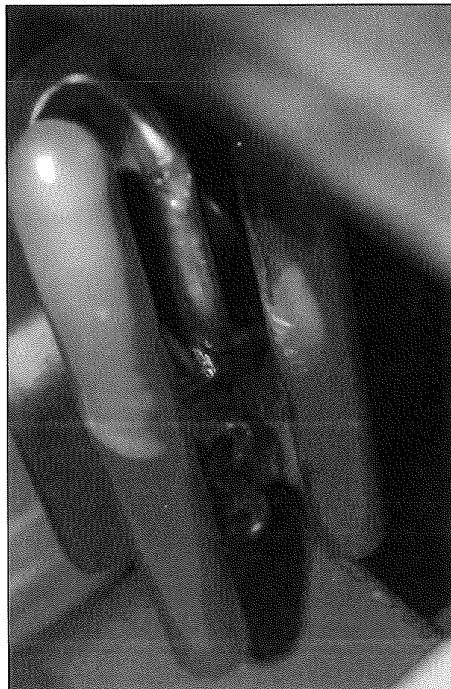
Photo No. 04 After PEHLA 08008Ra / 10 (fixed contact of phase L1, all contacts in comparable condition)
