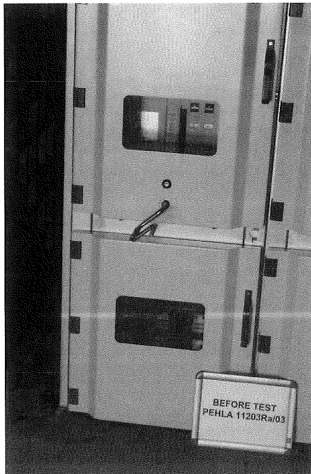
Photo No. 04 Before test PEHLA 11203Ra / 03
